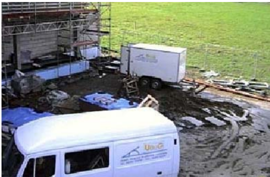
Figure 12: TRT-equipment of UBeG GbR on site for design of a BHE field in Aachen, Germany
