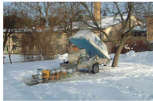
Figure 1: Swedish test rig, coupled to a borehole heat exchanger
